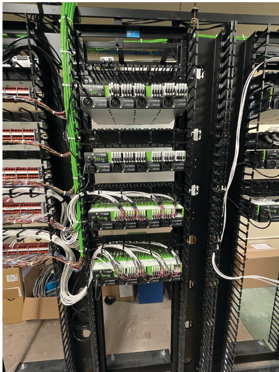
DIGITAL ELECTRICITY TRANSMITTERS IN THE MDF
